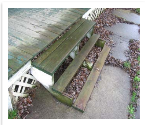
Damaged/missing treads and risers.
