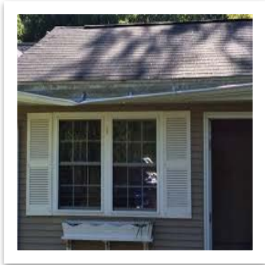
Section of gutter needs repair.
