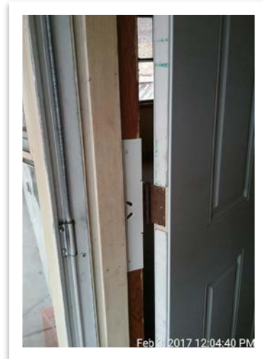
Photo showing door hinge protection product installed.
