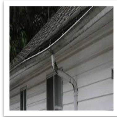
Section of gutter needs repair.
