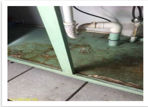
Chemical residue left under a sink.
