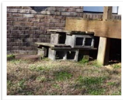
Unacceptable use of materials.
