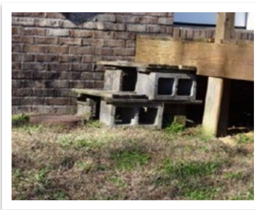
Unacceptable use of materials.
