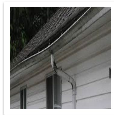
Section of gutter needs repair.
