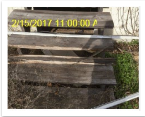
Damaged treads and risers.
