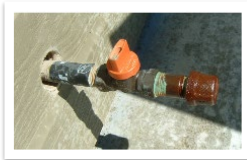
Gas line shut off and capped correctly.
