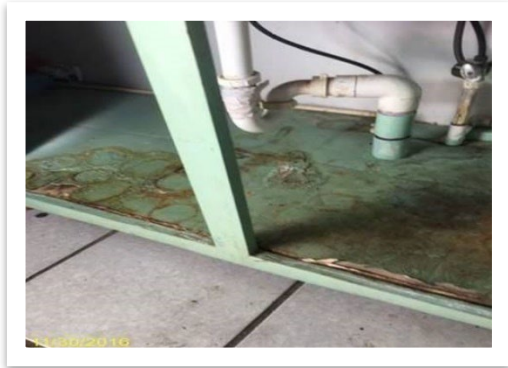
Chemical residue left under a sink.
