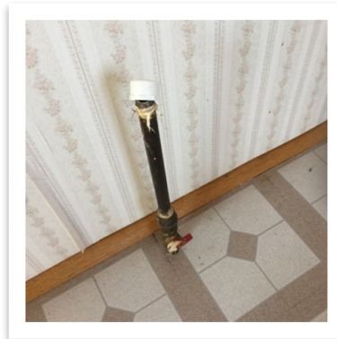
Incorrect type of gas line cap.
