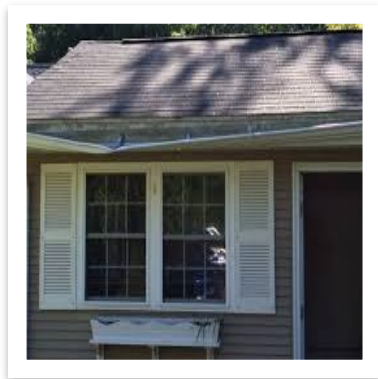
Section of gutter needs repair.
