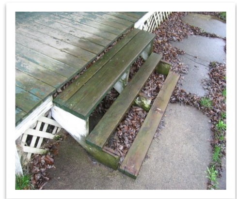
Damaged/missing treads and risers.
